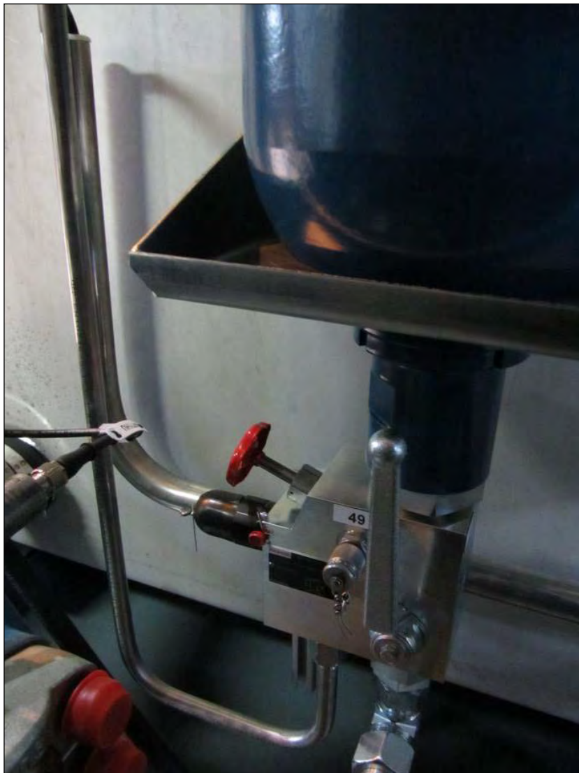
Figure 25. Discharge hand valve
