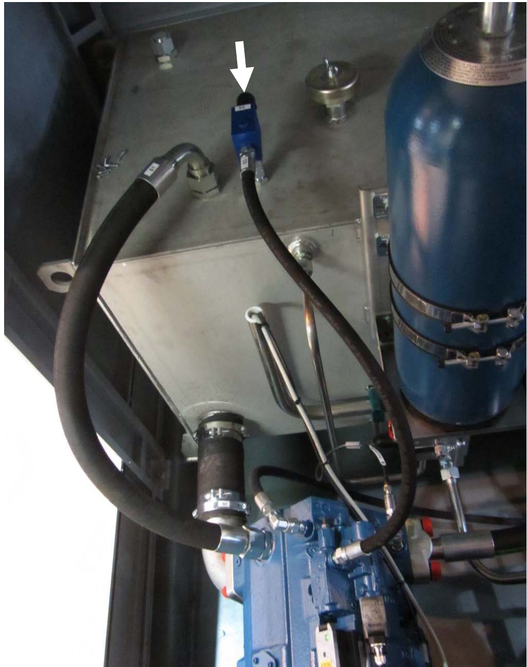
Figure 36. Pump P1 control pressure relief valve
