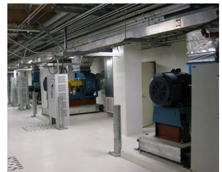
Exhaust Fans for Nuclear Plant
