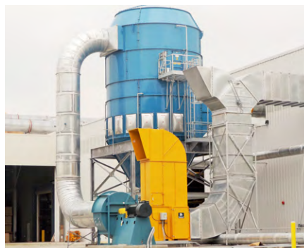
Dust Collection System
